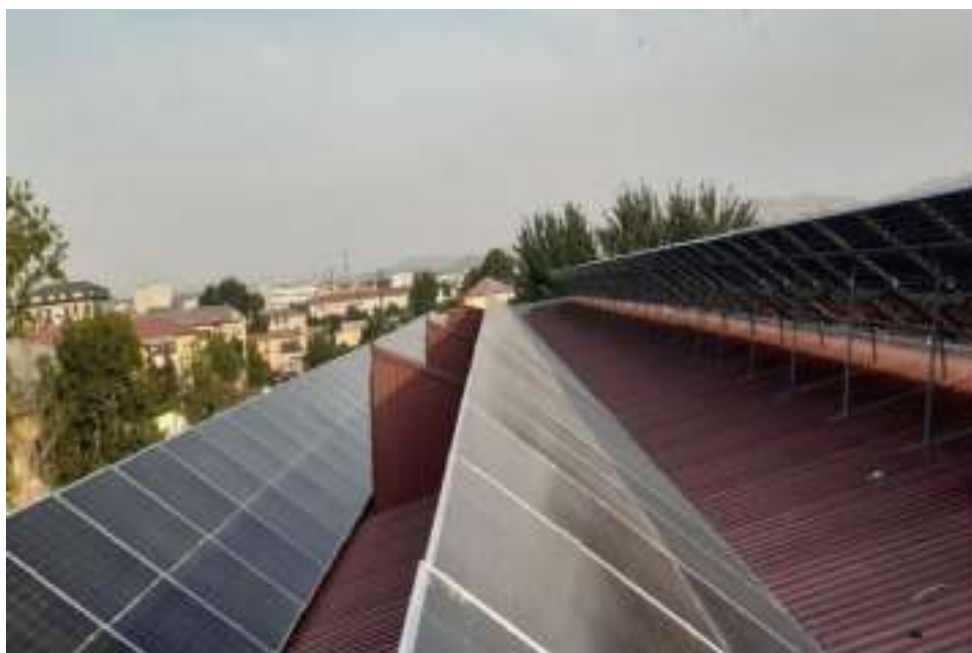
Fig.1.3: Solar power plant at the Andijan Mechanical Engineering Institute.
