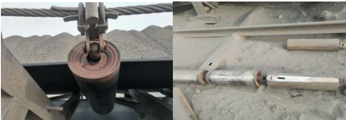
Figure 2. Belt conveyor rollers
